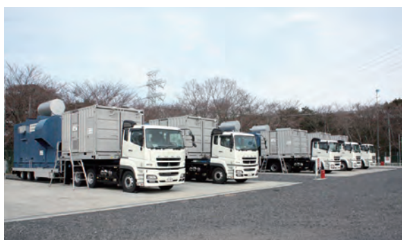
[電源容量: 1,725kVA(1台)×5台=8,625kVA]
